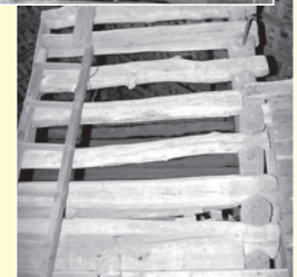
Log Construction Shows some of the original log construction inside the Bushman barn.
